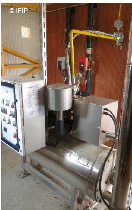
Chaudière biogaz / propane
